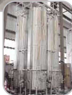
Water Reclamation Module, 500,000 gallons per day capacity.
