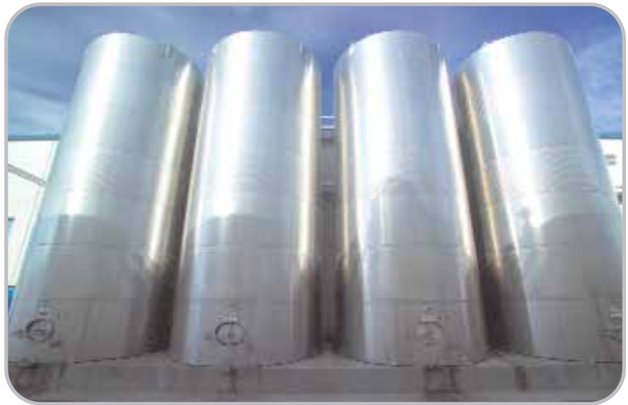
15,000 gallon Bulk Wine Storage Tanks, bench mounted for outdoor service.
