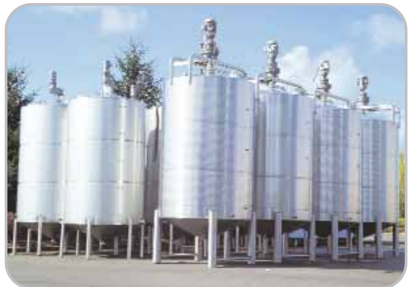
5,500 gallon jacketed Mix Tanks (for high viscous products), with scrape surface mixers and high efficiency gear motors/reducers (right). 3,400 gallon BioDiesel Reactors with explosion-proof mixer motors (left).
